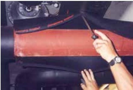
One of the first AF/ArmaFlex installations and still in operation.
